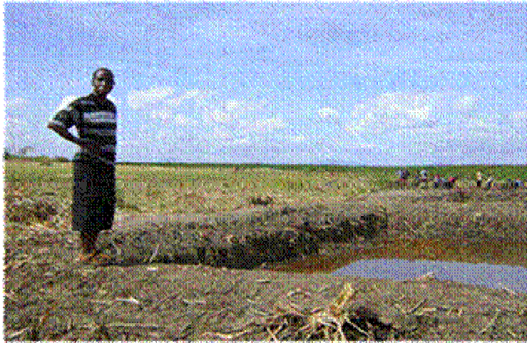
Figure 15. A member of the research team supervising ponds being constructed and compacted
