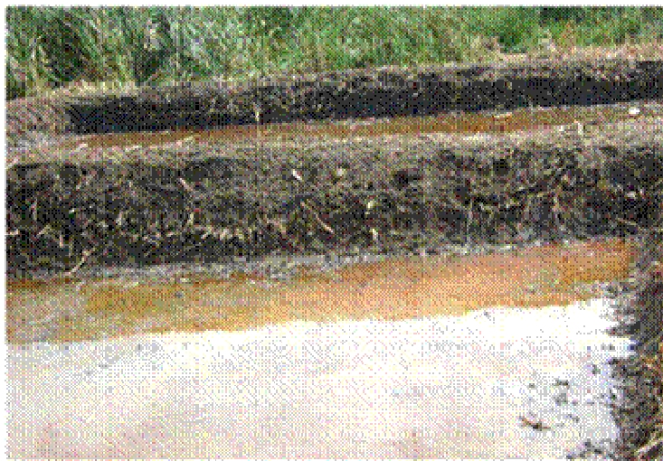
Figure 14. Two of the six ponds excavated being compacted and partly filled with water
