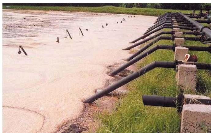
Multifunctional sewage treatment ponds at Webuye Pan Paper Industry. Photo: O. On'gan'a.
