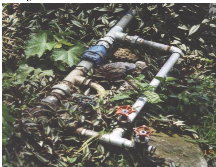
Figure 6-20: Pass by pipe (water metering)
