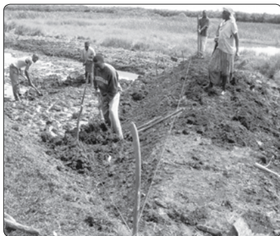
Figure 2.2-2. Pond construction typically involves excavating the inner area and using that soil to build the embankments.
