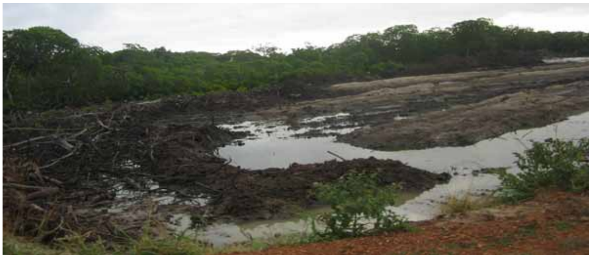
Plate 22: An extensive area of mangrove forest being cleared to give way to the LaPSSET Project infrastructure development (Photo: Onywere, Oct. 2015)
