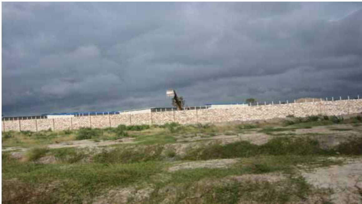
Plate 42: Massive construction site at Magogoni nere the site for the Lamu Port. (Photo: Onywere, Oct 2015)
