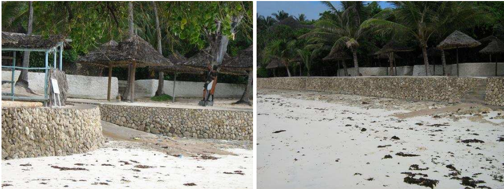
Figure 2: starting erosion and an elevated beach at Leopard Beach.
