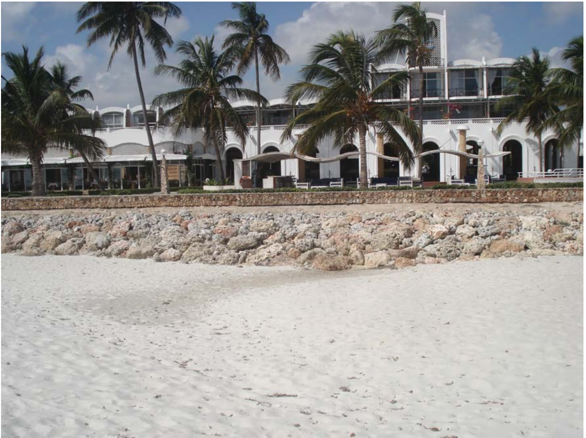
Fig. 36. Seafront hotel protected by a rock-block revetment and capping wall, Kunduchi site. Photo: Y.W. Shaghude.
