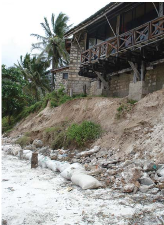
Fig. 38. A beach hotel threatened by erosion along the Nyali beach, Bamburi site, October 2007. Photo: J.W. Mburu.
