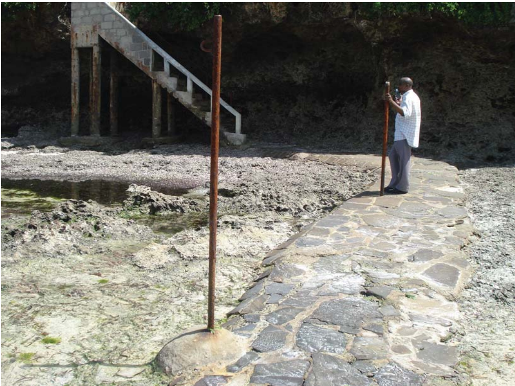
Fig. 13. Site of Beach Profile BP 00 at Nyali Beach, Bamburi site: ( Top) in April 2008 with an abundance of beach sand, and (Bottom) in February 2009 with an absence of beach sand against the base of the stairway. (Photos: J.W. Mburu).
