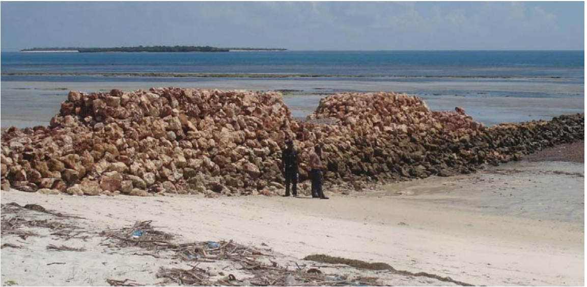
Fig. 48. Groyne constructed of quarried rock blocks on the Kunduchi shore between the Beachcomber and Whitesands hotels (see Fig. 49). Photo Y.W. Shaghude.
