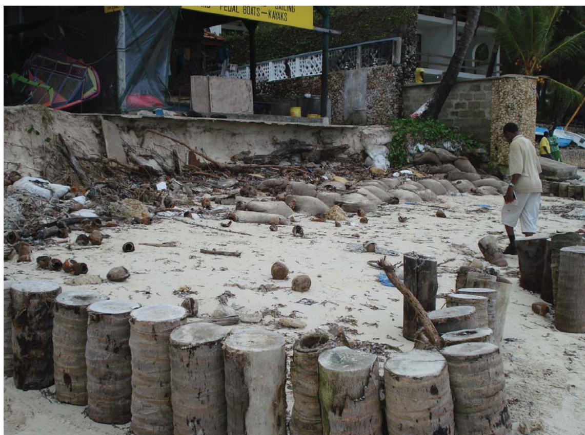
Fig. 1. Seafront buildings threatened by erosion, Bamburi study site, Kenya. Photo J.W. Mburu.
