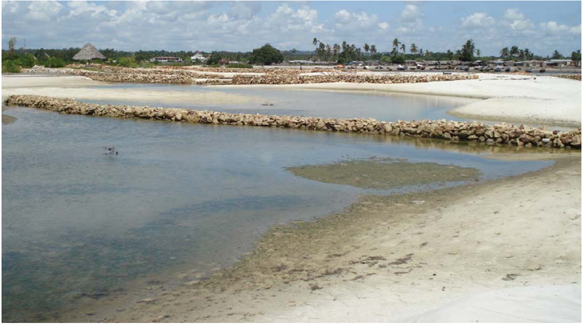
Fig. 50. Groynes comprising quarried rock blocks installed on the Kunduchi shore north of the Beachcomber Hotel, at the site of the former Africana Hotel (see Fig. 49). Photo R.S. Arthurton.
