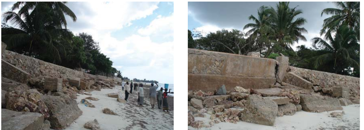
Fig. 47. Failing seawalls with block aprons between Kawe and the Mbezi River, Kunduchi shore. Photos Y.W. Shaghude.
