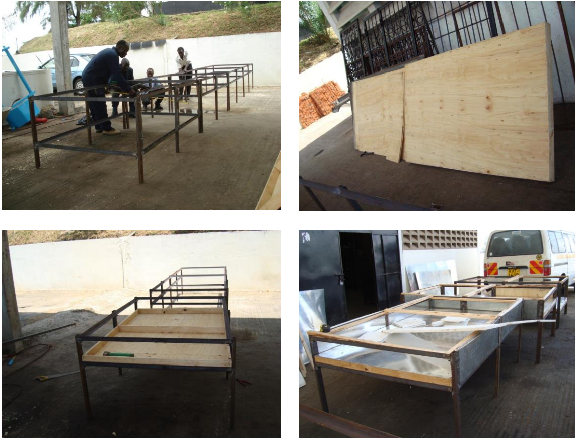
Figure 2.1: Construction of the main frame of collector for the hybrid windmill solar tunnel dryer with the boards and aluminium sheets
