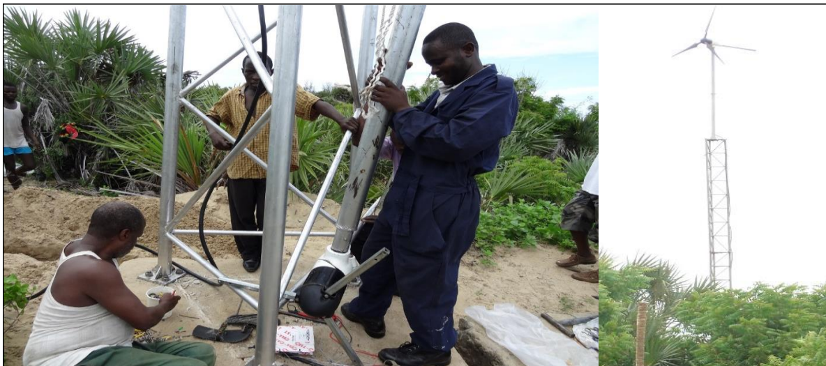
Figure 2.7: The wind generator about to be hoisted and the windmill in operation for the hybrid windmill solar tunnel dryer in Kipin, Kenya
