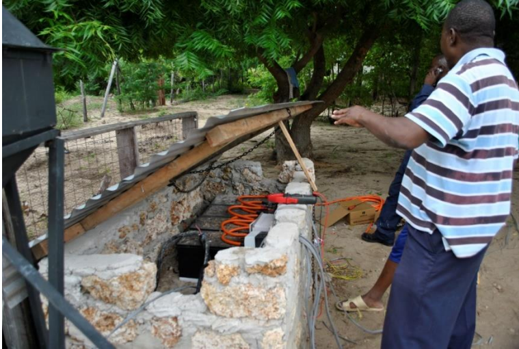
Figure 2.8: The battery bank and inverter for the hybrid windmill solar tunnel dryer in Kipini, Kenya
