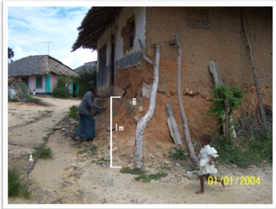
Figure 7.4: Signs of erosion in Jomvu village. The point marked B (Notice the man pointing) is claimed to be the ground level 50-60 years ago when the house was being built. The point marked A is a water pipe that is usually buried more than 1m below the surface. This pipe was installed in the 1960's (Photo taken during study in 2004).
